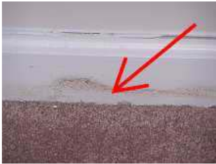
Photo 33 Water stain on base board.
