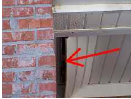
Photo 24 Siding coming loose on front porch.
