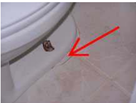
Photo 40 Tile cracked around toilet near floor.
