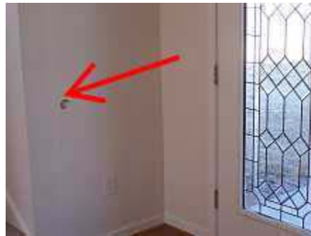
Photo 38 Hole in wall from front door. No door stopper installed.
